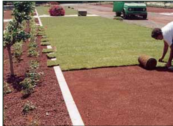
Installation of roll grass on a base of volcanic aggregate with grain size 0 -12 mm.
